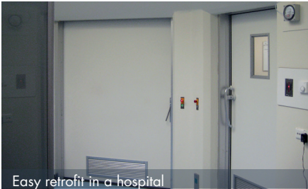
Easy retrofit in a hospital
