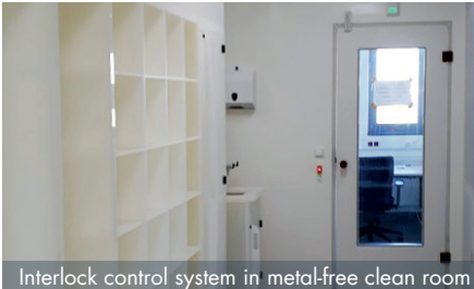
Interlock control system in metal-free clean room
