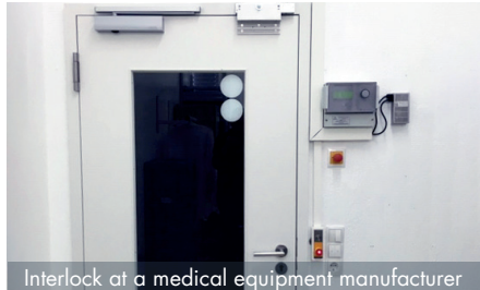
Interlock at a medical equipment manufacturer
