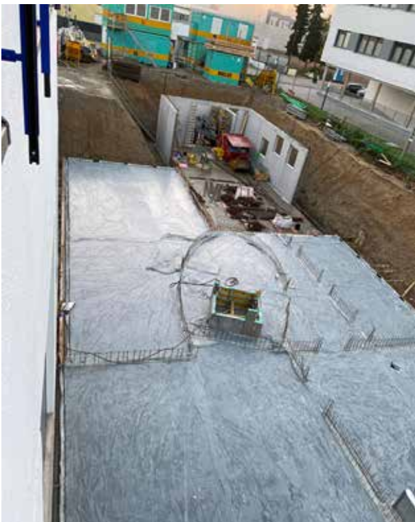
The complete base plate is ready. The first outlines are visible. The characteristic ellipse of the new building can be seen in the center. This is where the stairwell is being built.
