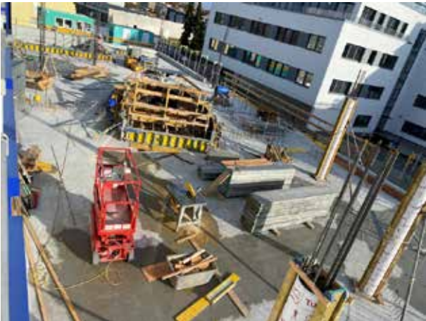
In the front area, the supports have not yet been boarded up.
