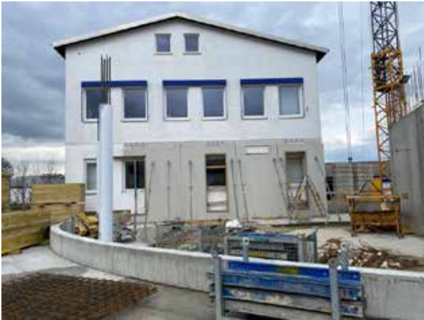
And already we are on the 1st floor. In the south facade of the old building, 2 windows have already disappeared behind a concrete wall. The later connecting doors are already clearly visible in the boarding.
