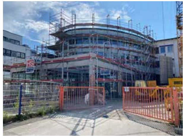
Most of the facade elements are already in place - but the many seals are still missing.
