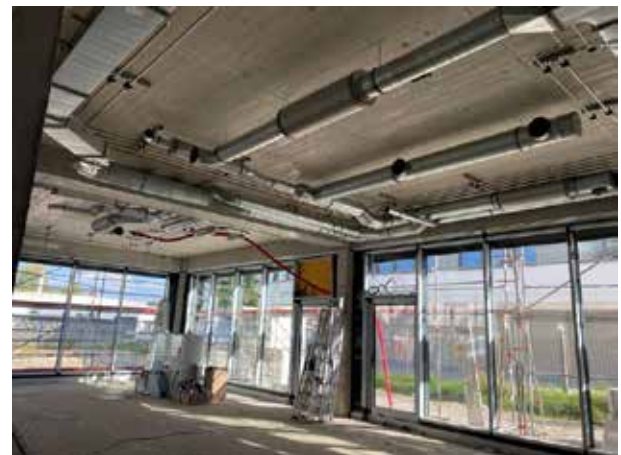
Ventilation pipes are now also already being laid in the multifunction room
