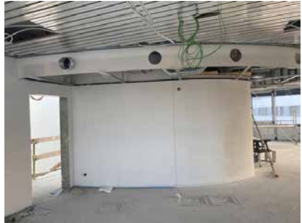
The holes in the upper cladding are for the air vents of the ventilation system.
