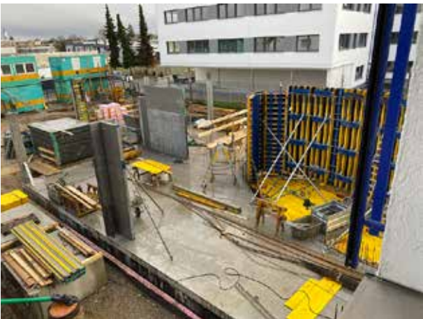
The first columns for the large seminar and conference room are now in place (top left).
