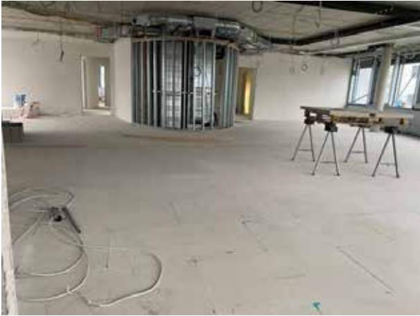
The floor is finished. Now it's time to cover the ventilation ducts and pipes that run along the stairwell ellipse from the basement to the second floor. The stud frame is already in place.
