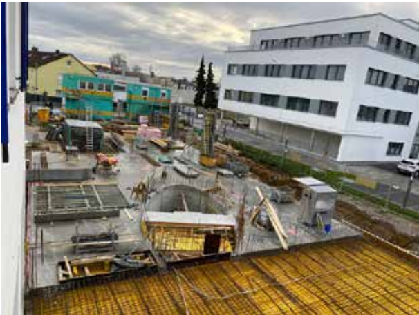
After the winter break, work continues at full speed in the front area. Only the back warehouse area is still waiting for the heating loops to be laid. Nice to see: the elliptical stairwell with the "bridge" leading from one side to the other.
