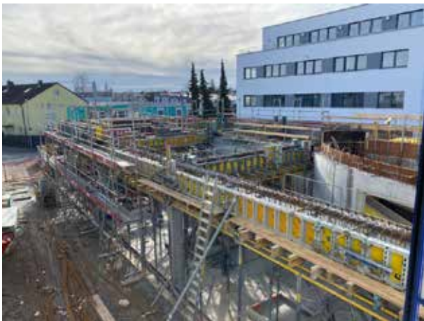
The beams have been concreted. Now their formwork must be removed so that the slab formwork can be placed in this area as well.
