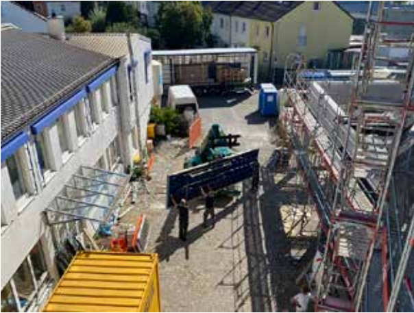
The almost 7 m long side sections of the stock storage machine have to be transported to the installation site – no easy task.
