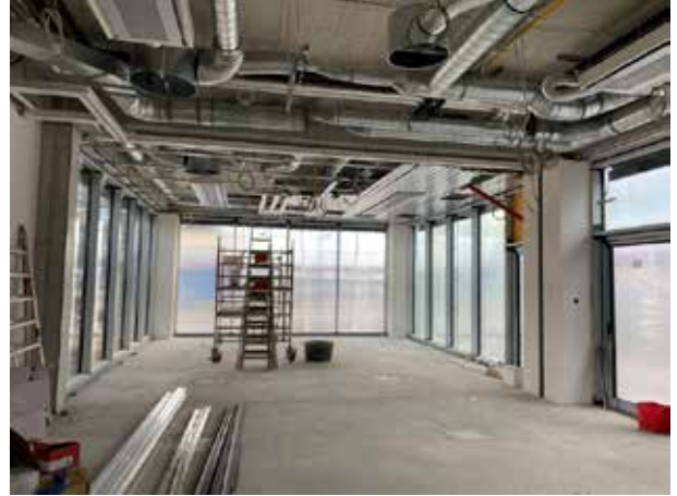
Work is still underway on laying the heating/cooling ceiling in the multifunctional area.
