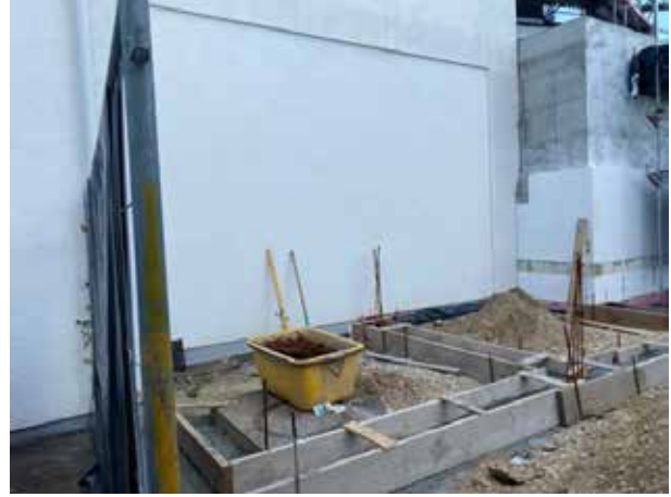
Behind the building, a small annex is being built as storage for trash cans for clean trash separation, as well as a separate room for gardening tools, etc.
