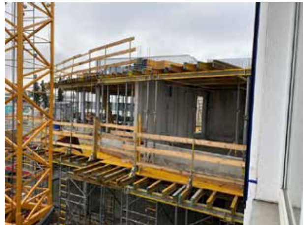
And the construction work continues: on the 1st floor, the ceiling boarding is being installed.
