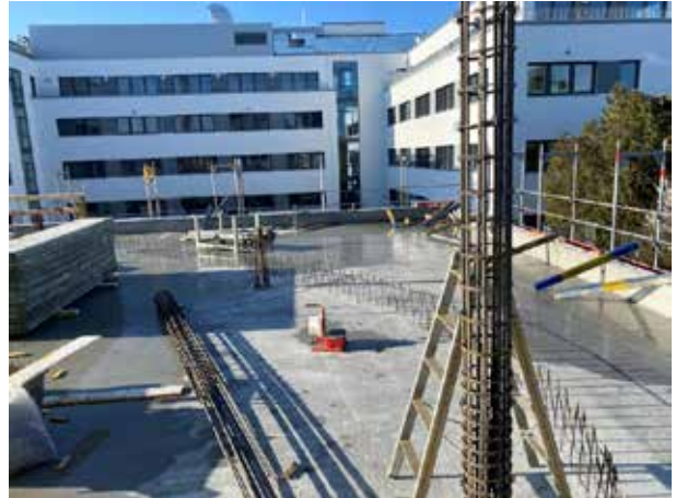
Next, the columns that support the ceiling of the 1st floor are created.
