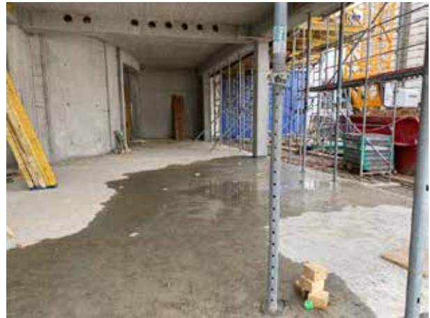
Another tour is due: the entrance and exhibition area on the first floor – now already without supports.
