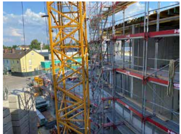
View from the 2nd floor of the old building to the extension.
