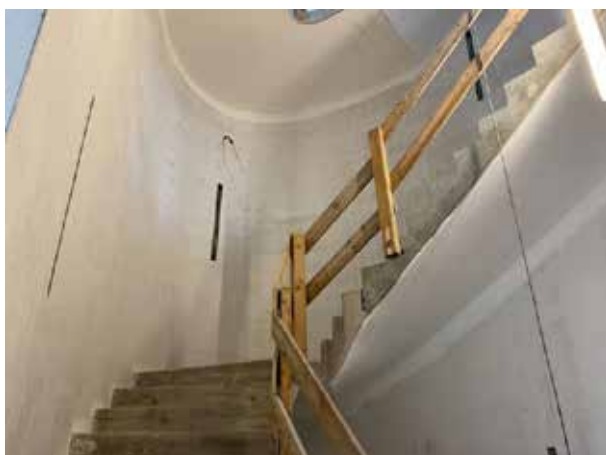
The stairwell has been plastered – and you can use the stairs to get to the upper floors again.
