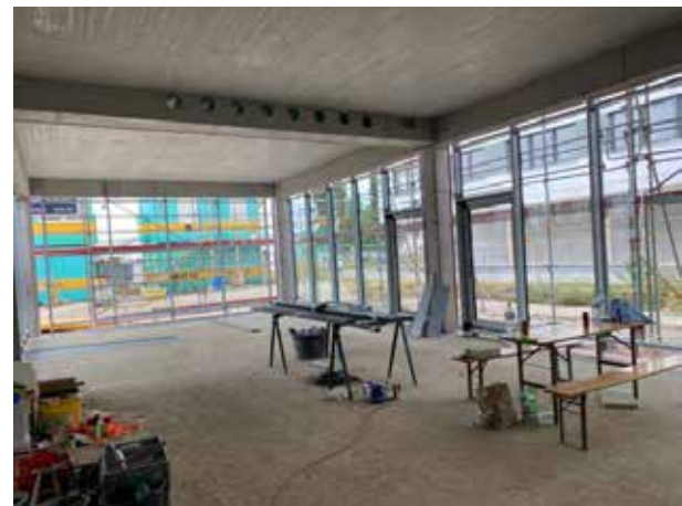
Our multifunction room on the first floor. So gradually you can imagine the appearance a little better. A mobile partition in the middle allows the room to be divided into two independent rooms.
