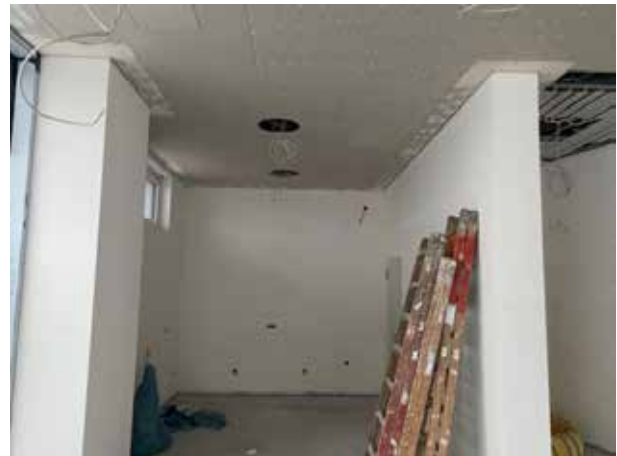
There will later be a kitchen here so that guests can also be catered for at events in the multifunctional room.
