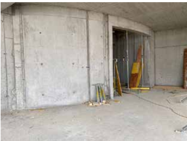
We walk towards the staircase, which will later be as bright as the other rooms – through a glass dome in the roof.
