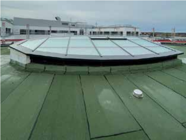
To see the glass roof from the outside, you have to climb over the outer scaffolding up to the roof.
