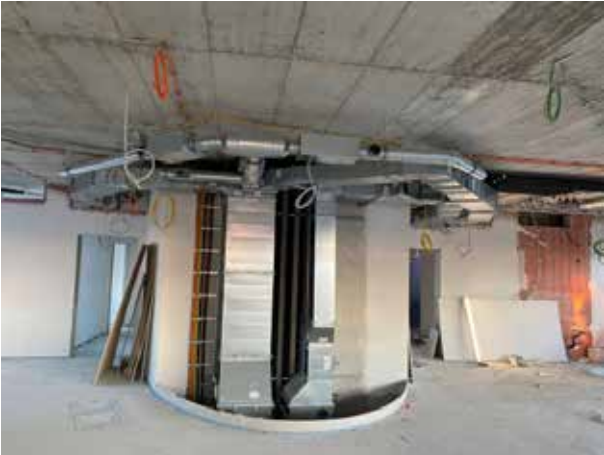
The ventilation ducts & pipes on the 2nd floor. The ventilation ducts for the open-plan office can be seen on the ceiling.
