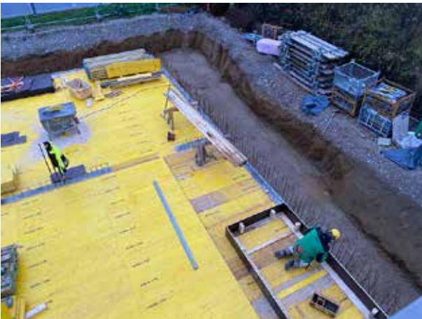
The passage in the basement ceiling to the first floor is being formed. This is where our automatic storage system will be located later on – so that we always have enough space for sufficient stock and can deliver quickly.
