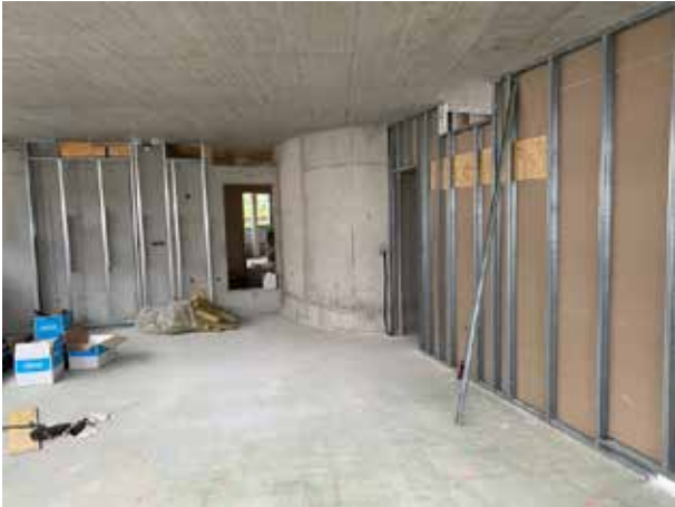
Drywall is being installed on the 1st and 2nd floors. This is the future lounge – photographed from the exit to the roof terrace.
