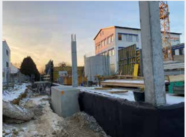
View from outside into the training and conference area. No exterior walls will be concreted here; instead, there will only be concrete columns, between which glass walls will provide an open feel.
