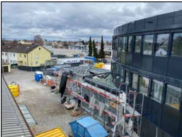
The steel structure is in place. The glass roof now needs to be drained before the glass panes are installed.
