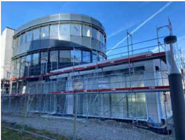
The scaffolding is still up on the first floor. Here, the outer façade (everything around the windows) still needs to be insulated. The glass windows covered with plastic belong to the multifunction room.
