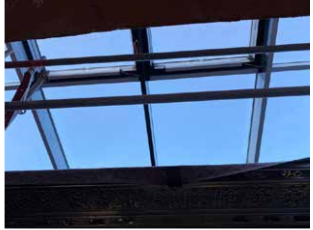
You can't yet see the glass roof in all its glory from the inside, as there is scaffolding underneath it.
