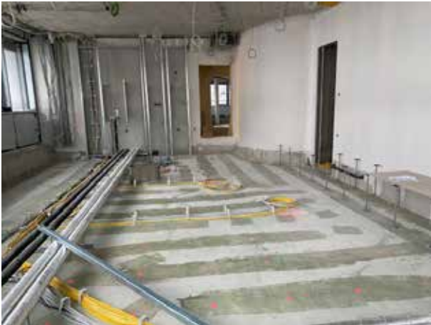
The false floor will be installed in the future lounge. The supports look pretty thin at first glance – but they hold.
