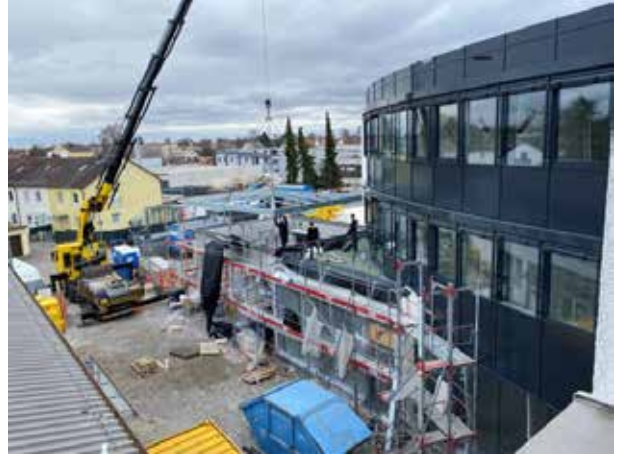
A large glass roof will be built over the entrance area so that everyone who comes to us will also find a dry place in front of the building. The steel construction to hold the glass panels is "flown in".
