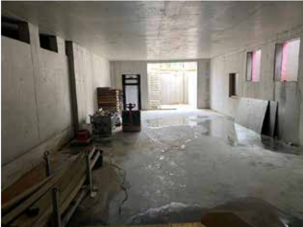
This basement was built exclusively for the ventilation system. The new building should not be spoiled by vast amounts of technology on the roof.
