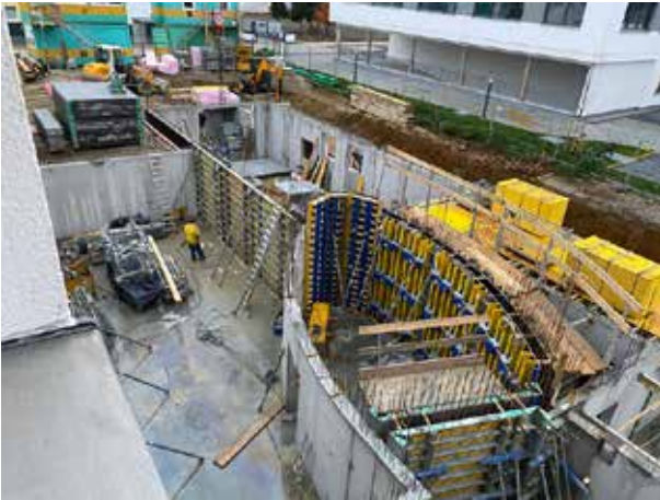
The remaining interior basement walls are formed – ready for the concrete to be poured.
