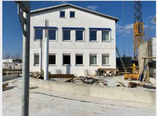
And now we are on the first floor. In the area outside the interior base, a green rooftop area will be created. A beautiful view for everyone in the future sales office.
