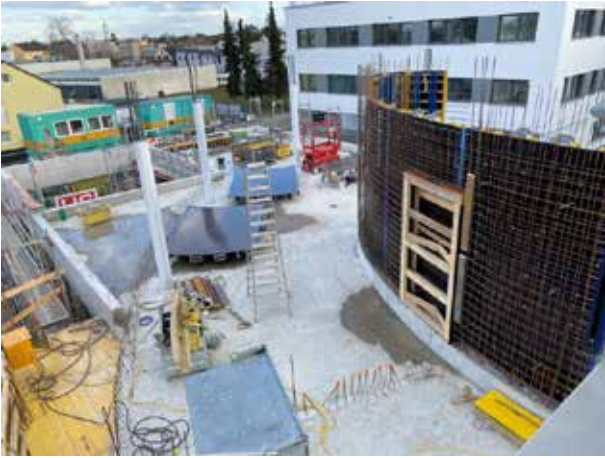
You can clearly see where the opening to the staircase will be later on. The area to the left of the two columns outside the ellipse will become a small terrace for the meeting room. At the very back, the roof terrace in front of the staff lounge can be seen.
