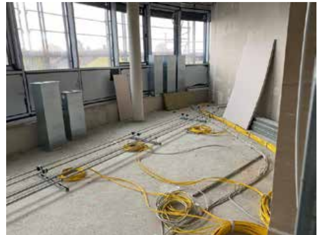
More pipes and cables are still being laid on the floor on the 1st floor.
