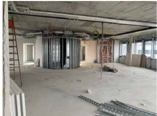
This is where the technical customer service department will be located. The studwork for cladding the ventilation ducts and pipes around the stairwell ellipse is already in place.
