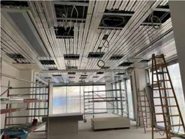
The heating and cooling ceiling and the ventilation units are installed in the multifunctional room.
