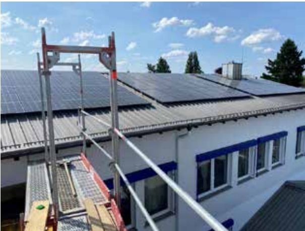
The photovoltaic system on our existing building. On the sunny, long days at the end of May 2023, we are self-sufficient in our power supply – and even supply electricity to the grid.
