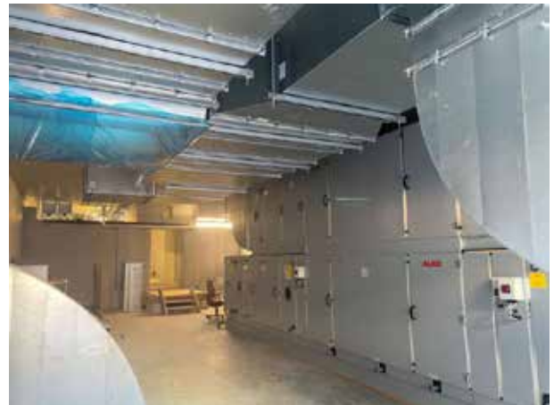
The ventilation cellar is now packed with the plant and ventilation ducts
