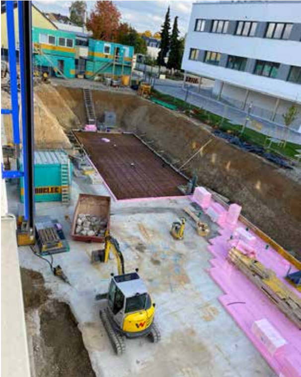
The only thing missing is concrete in the front basement area.
