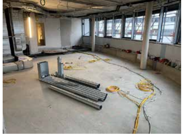
There is no screed on the 1st floor, as a double floor will later cover all the pipes, ducts and cables on the floor. Here too, the heating/cooling is laid in the ceiling.
