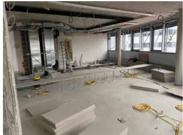
And now the false floor is also being installed in the open-plan office, where our internal sales team will be there for you later. At the moment, it looks more like a catwalk!
