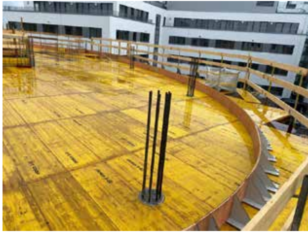
The elliptical formwork for the ceiling of the 1st floor is created...
