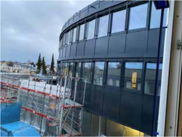
On January 24th, the time has come: the scaffolding for the 1st and 2nd floors is removed.
