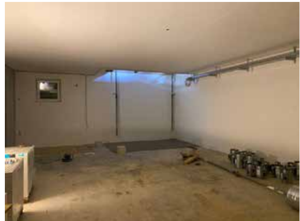
This is where the stock storage machine will be located – although this is only a view of the first floor. It will extend over two floors: basement and ground floor.
