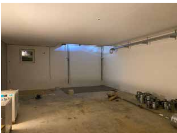
Here will find its place our storage vending machine, which goes over two floors (basement and first floor)
