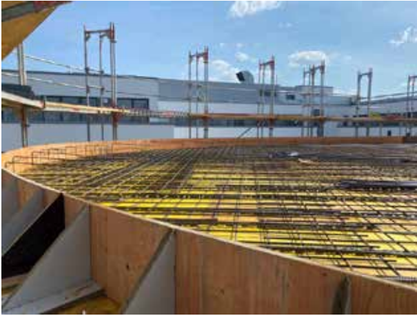
The boarding of the ceiling of the 2nd floor – almost looks like a work of art.
