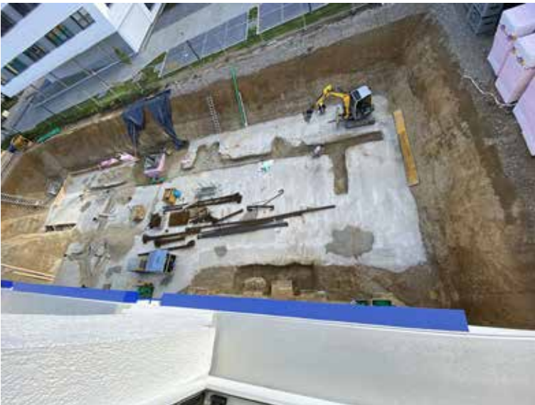
The sump is already isolated.
