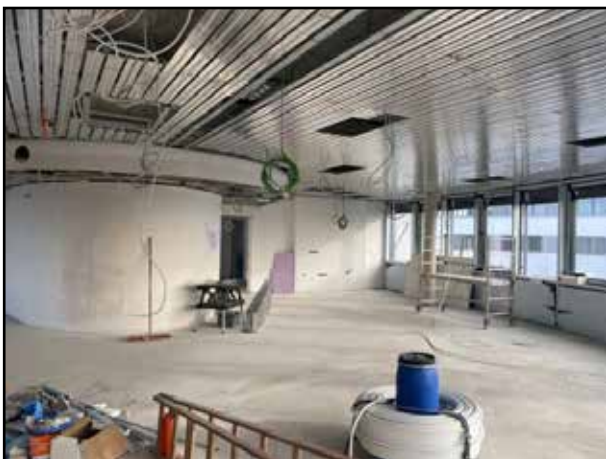
A small kitchenette will be located on the wall at the back right.
