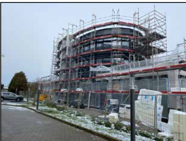
The exterior was plastered and painted, just in time for the onset of winter.
