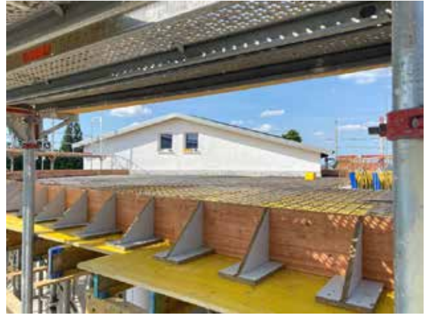
Another view of the existing building. The window sills of the skylights serve as a shelf for the steel weavers.
