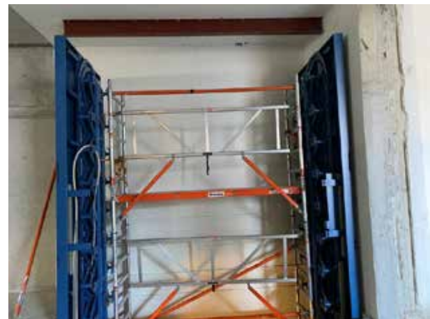
Scaffolding has been erected for the rest of the assembly work – here is a view of it on the ground floor.
