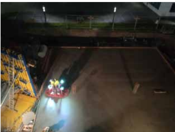
On January 18th, the warehouse floor is concreted despite low temperatures. The concrete polisher works until late in the evening – certainly no fun at temperatures around freezing point.
