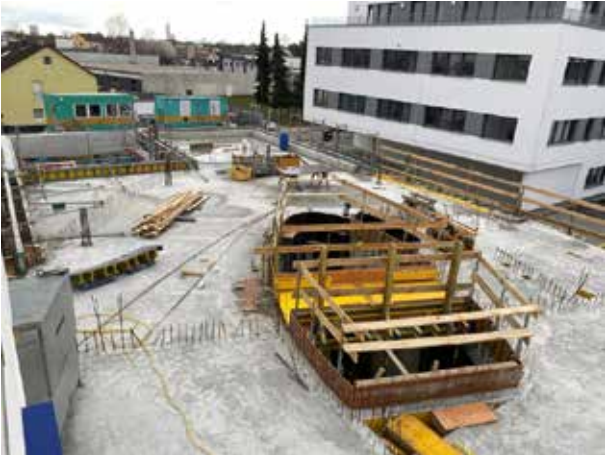
And work is already underway again on the formwork for the staircase ellipse . The first thing to be created is the "bridge".
