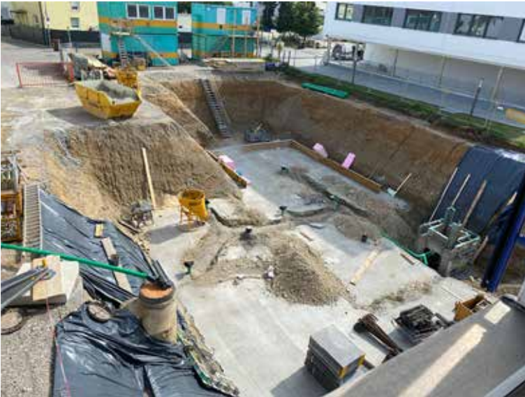
The wastewater pipes are laid. For this purpose, the subbase must be partially removed. Hammer drills and excavators are a background noise in everyday office life.
