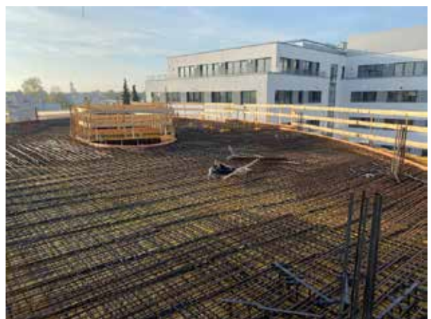
..... until you can no longer see the formwork boards because of all the structural steel. But now everything is ready for concreting.
