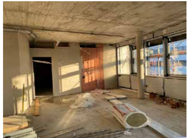
On the 2nd floor, only screed is applied to the floor, so that the ducts for the electrical installation on the floor are not allowed to be too thick. The first walls are plastered.
