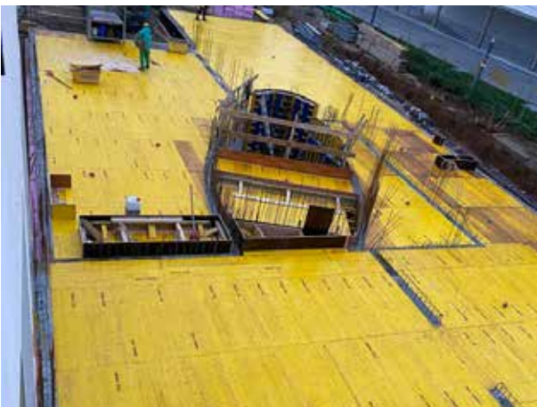
The casing for the entire basement ceiling is finished. In the ellipse, you can see the "bridge" that takes you from one side of the stairwell to the other. Now it's the steel weavers' turn.
