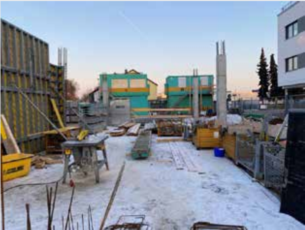
Here will be a storage room and a kitchen for the training and conference rooms in front.
