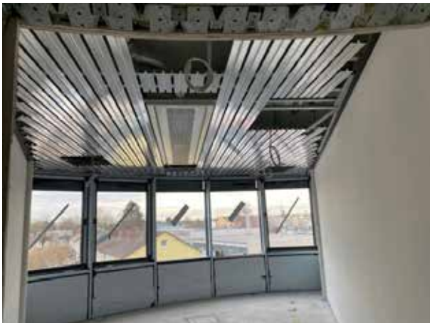
There are several smaller offices on the 2nd floor. The heating and air conditioning ceilings with the ventilation systems are currently being installed here.
