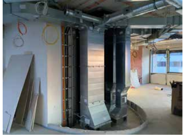
Until recently, the openings between the floors near the ventilation ducts were still open. Now they are sealed off to protect against fire.
