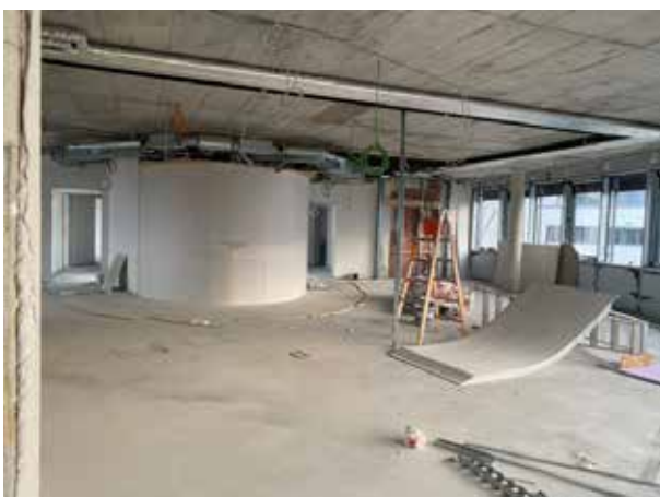
And now a large part of the cladding has already been fitted. Note the "device" for bending the panels.
