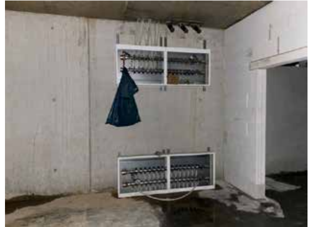
The first signs that in this basement room will be installed heating. We work environmentally friendly with a heat pump.
