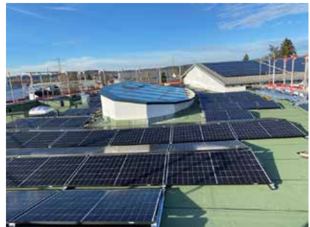
The weather is kind in the last week before Christmas: the photovoltaic system can still be installed.
