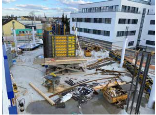
One side of the staircase ellipse and part of the base are ready for concreting.
