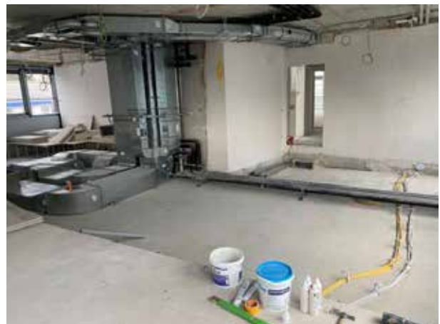
In the front area, the ventilation ducts still have to disappear under the floor.
