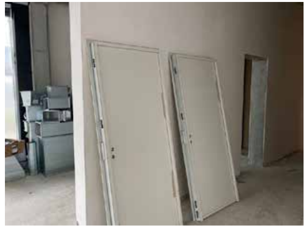
And the fire doors are also being installed. They are still waiting to be installed on the first floor.
