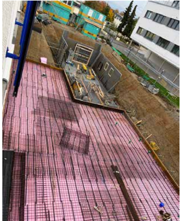
The steel braiders are hard at work and in the front area the casings for the first basement walls are being erected.
