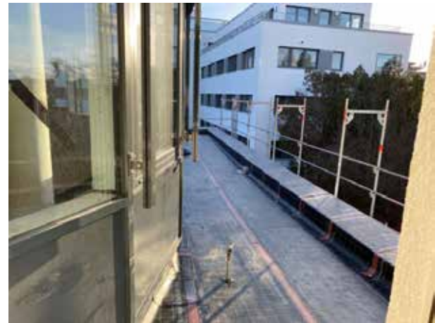
A green roof is being built on the roof of the first floor in the rear area. The first layer of tarpaulins has been laid.
