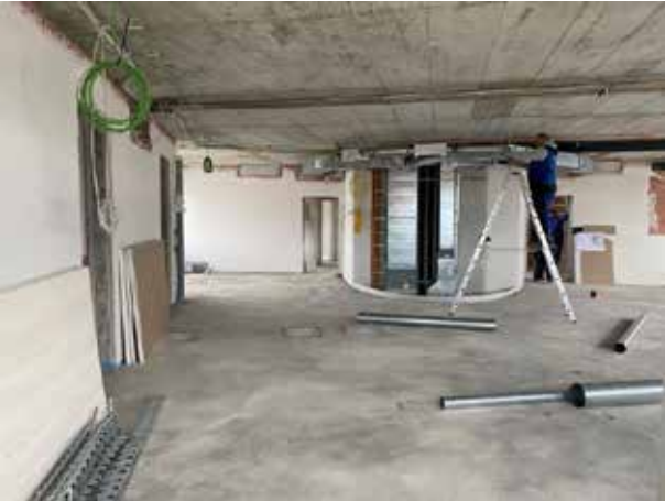
The screed has also been laid on the 2nd floor. The pipes for the heating/cooling run along the ceiling.
