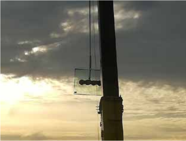
The glass panes for the glass roof above the stairwell fly in. They are not hanging by a thread, but by glass suction cups – but they hold.
