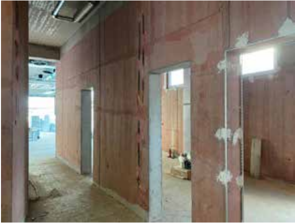
All the concrete walls on the first floor have also already been primed.
