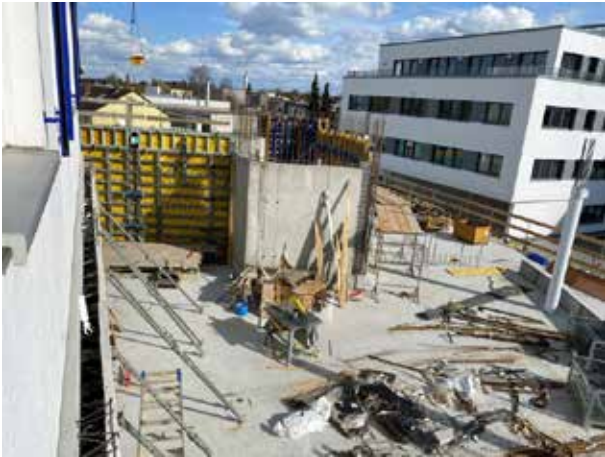
After the staircase ellipse is formed on the second floor the first wall...
