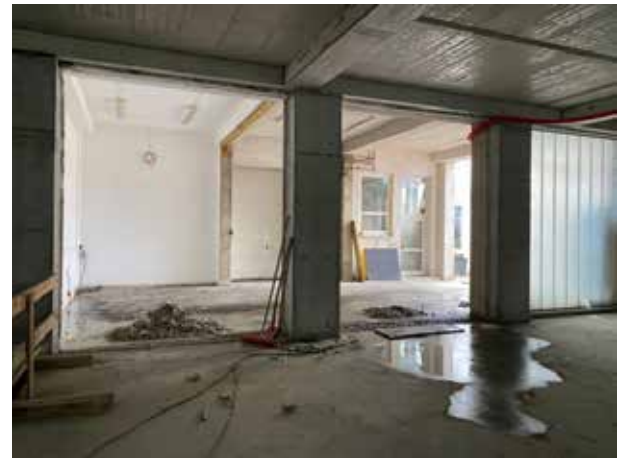
The connection of the new warehouse to the old building is open except for an old wall element that still has to be removed. Subsequently, the old tar pavement still has to be broken out and a new floor slab has to be created.
