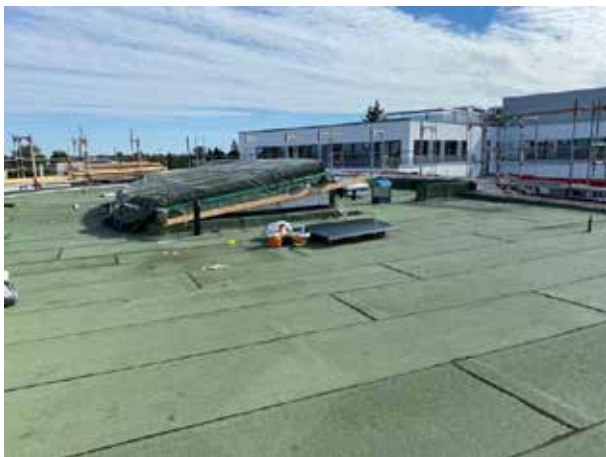
The glass panes are still missing, so the frame construction had to be wrapped again to make it weatherproof and rain-proof.
