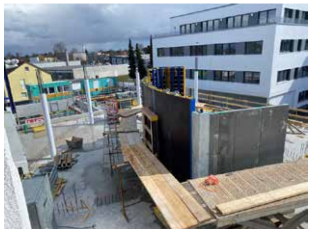
The outlines of the stairwell ellipse on the 1st floor are already visible through the formwork. In the meantime, the columns in the front area have also been concreted.
