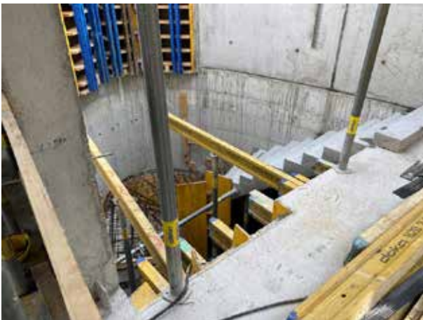
What you can't see from the old building is the work on the staircase. One part is done with prefabricated elements, the remaining steps and landings have to be concreted on site.
