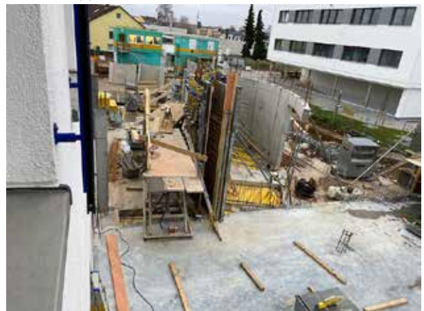
Another view from behind into the future stairwell. There is only one spot where the exterior formwork is still missing, so that concreting of the staircase wall can soon begin. The ground floor is taking shape and soon the construction site photos will probably have to be taken from the 2nd floor of our old building.
