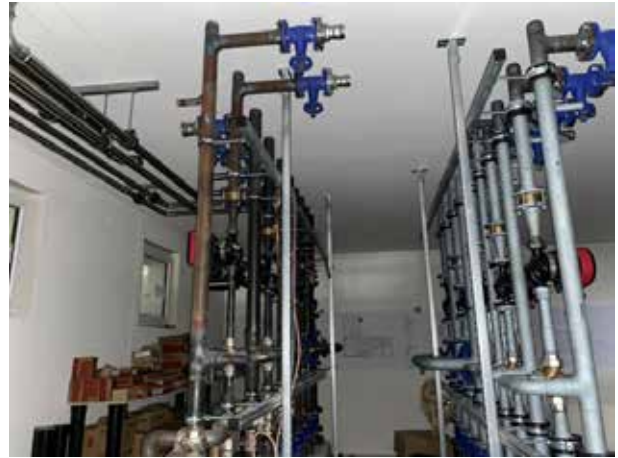
The distribution station for heating and cooling continues to expand.
