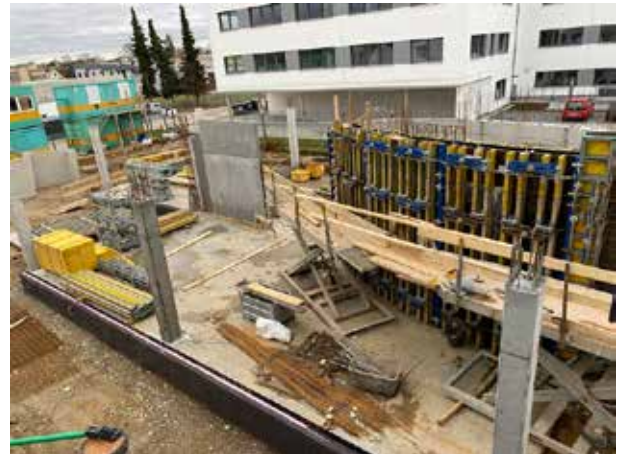
At the end of the week, the formwork on the other side of the staircase is almost finished. In the front area of the building, the first floor as well as the floors above will get a glass facade, which invites to come in. In the front of the picture you can see the future entrance area, where our visitors will find a showroom with information about our products and their areas of application.
