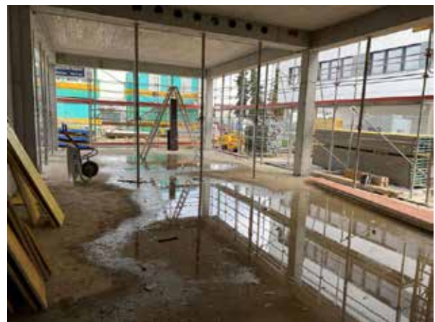
On the other side on the first floor is the meeting and event room – still a bit of a damp squib for visitors.
