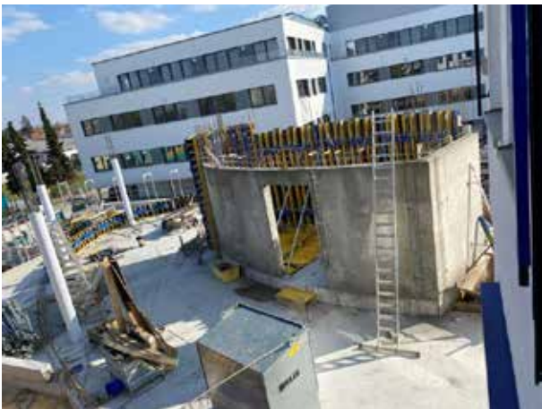
And already, on the 1st floor, the wall of the staircase is on one side – and the other is boarded up.
