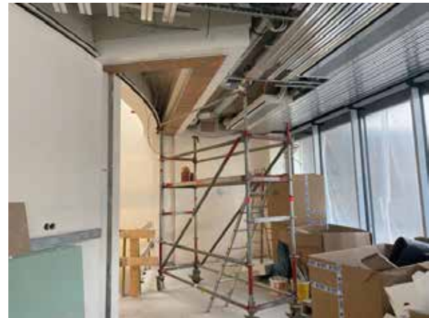
In the entrance area, the final ceiling is still missing in the rear area. The fire protection curtain in front of the stairwell still needs to be installed there.
