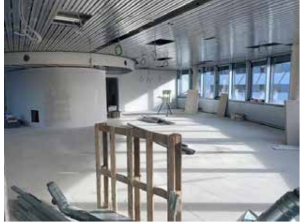
And now everything is clad. The heating and cooling ceiling has now also been installed. The office is taking shape.
