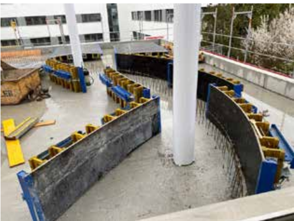
The outer base of the ellipse on the 1st floor is being boarded up. Between the ceiling of the first floor and the actual floor of the 1st floor there is space for electrics and other supply lines.
