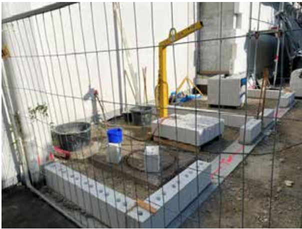
The walls of the extension are bricked - but the roof was then concreted again (for fire protection reasons).
