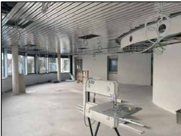
Where windows can still be seen at the back, the new building is connected to the old building by doors.
