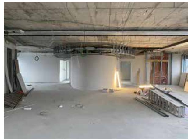
The cladding for the ventilation ducts is now also being installed on the ceiling around the ellipse.
