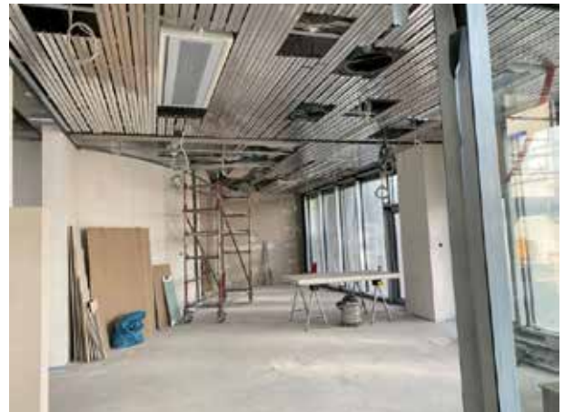
Another view of the entrance area from the front door. This is where an exhibition of DICTATOR products will be located in the future.
