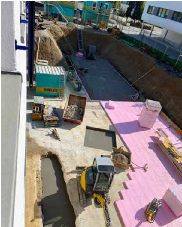
The rectangular shaft pit for the future DICTATOR DHE elevator can already be seen in the middle. 200 mm depth is enough.
