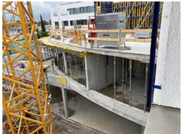
View from the 2nd floor of the old building to the extension.
