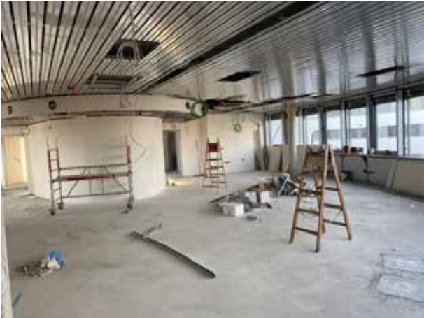
The air-conditioned ceiling is now also being installed in the open-plan office on the 2nd floor.
