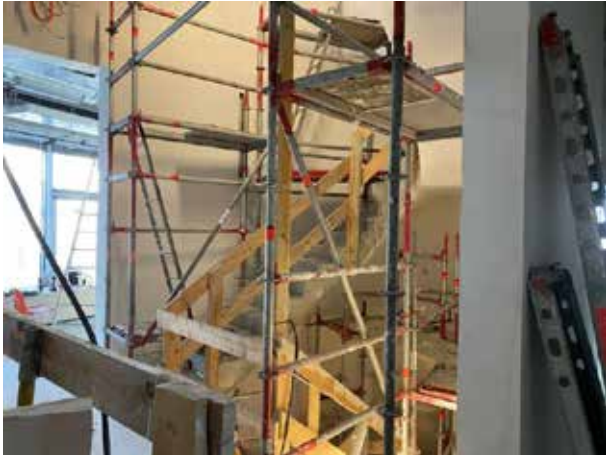
The stairwell is temporarily impassable as scaffolding has been erected for plastering.
