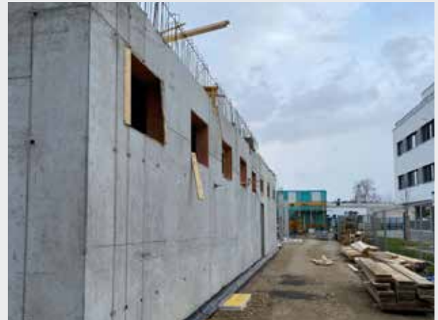
The bearing wall from the outside. During the week, the excavation pit was backfilled here as well. Scaffolding will be erected here shortly.
