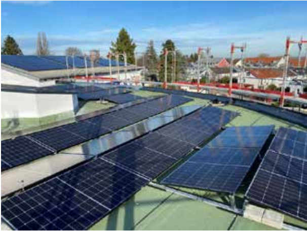
Photovoltaic systems are now installed on both roofs. This means that renewable energies play an important role at DICTATOR and contribute to improving the ecological balance.
